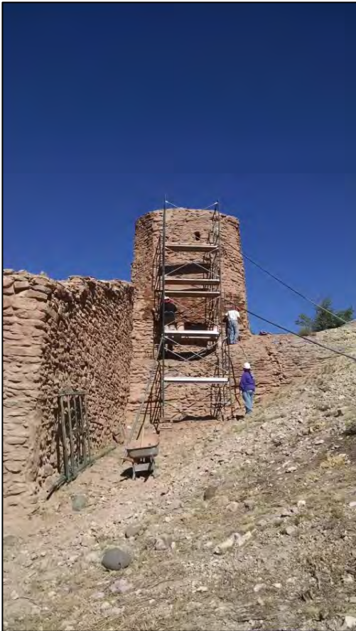
Work crew stabilizes the bell tower ruins at Jemez Historic Site. Photo by Matthew Barbour, courtesy of New Mexico Historic Sites.
